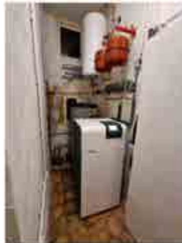
Figuur 9: water-water warmtepomp in woning
